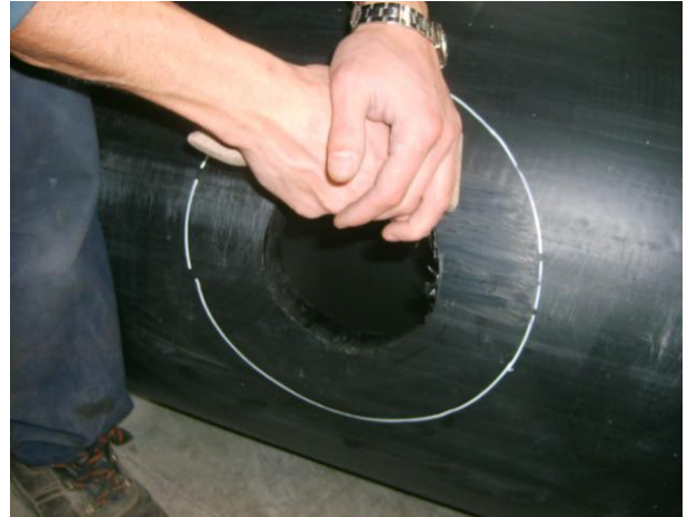
REMOVE OXIDE LAYER & ANY FOREIGN OBJECTS BY SCRAPING BETWEEN THE INTERIOR OUTLET HOLE & FUSION ZONE
