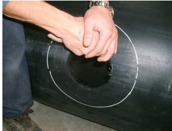
Scrape the thick field between interior and exterior circle to get the oxide layer on the pipe.
